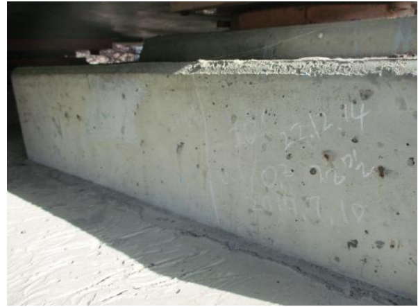
P3 Sh2 받침콘크리트 균열( Cw=0.1\text{mm}/0.3\text{m} )
